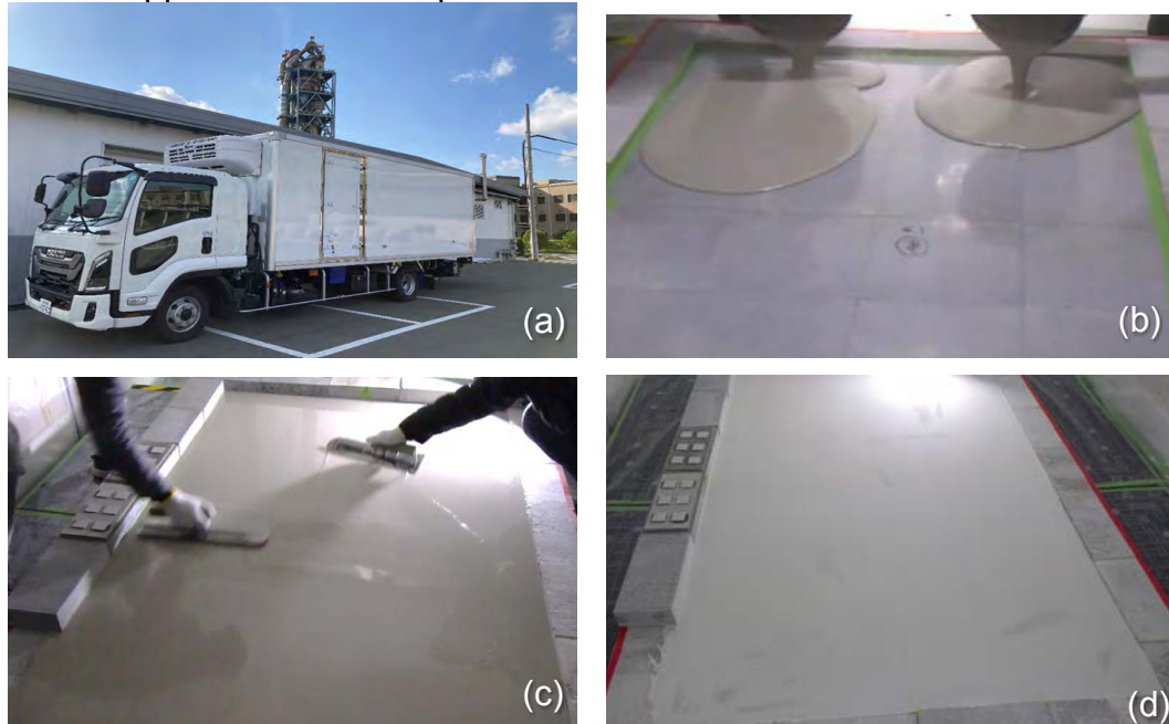
Figure 3. Field application trial inside a refrigerated truck at -25\text{ }^{\circ}\text{C} : (a) test environment (refrigerated truck), (b) mortar slurry placement, (c) troweling operation, and (d) finished surface without external heating.
